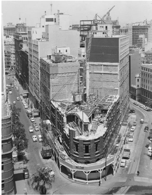
20 Demolition of the CSR Headquarters to make way for Knox House at 1 O'Connell Street Sydney Source: City of Sydney Archives
